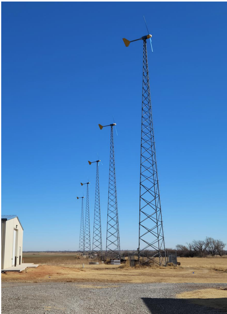
(5) Bergey Excel's on 100' Towers in Drummond, OK
