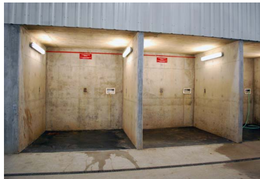
Confined wash stalls with internal floor drain and external trench drain
