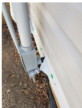
The wire is coming out of the house & into conduit going up to the meter. Nothing is protecting the wire or the wood it passes through in the house.
