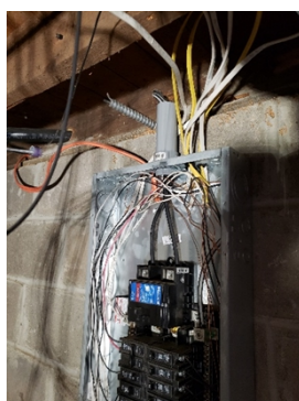
The panel does not have conduit all the way to the meter. The service wire is fanned out of the end of the conduit stub above the panel.
