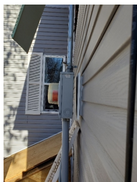
This meter socket is not attached to the house.
