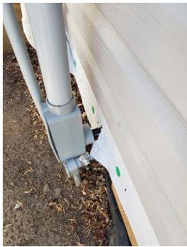
The wire is coming out of the house & into conduit going up to the meter. Nothing is protecting the wire or the wood it passes through in the house.
