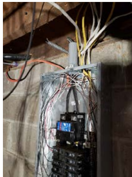
The panel does not have conduit all the way to the meter. The service wire is flown out of the end of the conduit stub above the panel.
