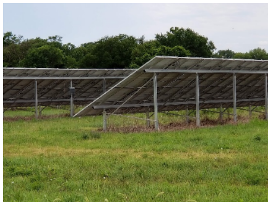
Example of a Solar Conversion System, Ground-mounted
