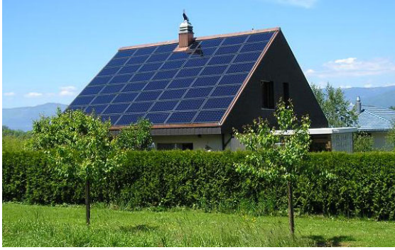
Example of a Solar Conversion System, Structure-mounted
