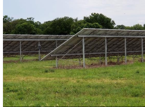
Example of a Solar Conversion System, Ground-mounted
